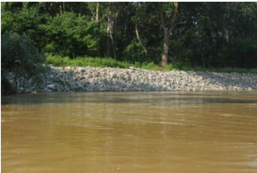
Figure 21: Continuous bank revetment by rip-rap (© Darko Grlica).
